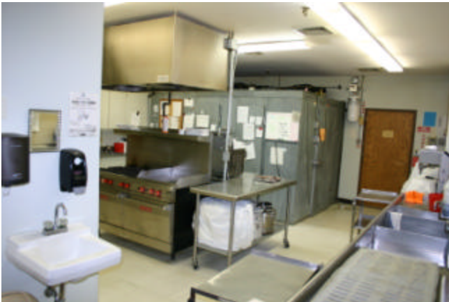
Photo 12 – Improve the kitchen work area and replace the walk-in cooler/freezer.
